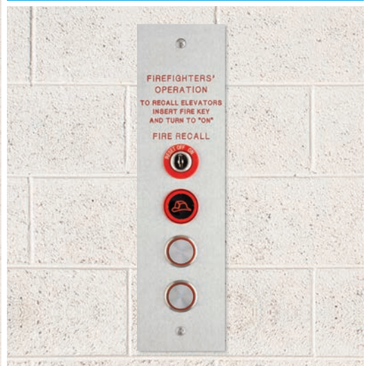
Intermediate hall station With fire services devices
