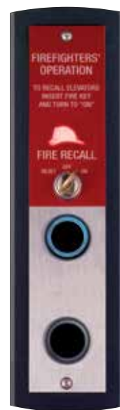
Combination hall station and fire service keyswitch (2004 code)
